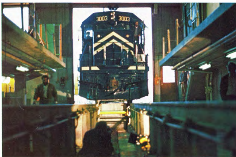
Little Rock repair shops perform preventive maintenance on up to 100 locomotives a day.
