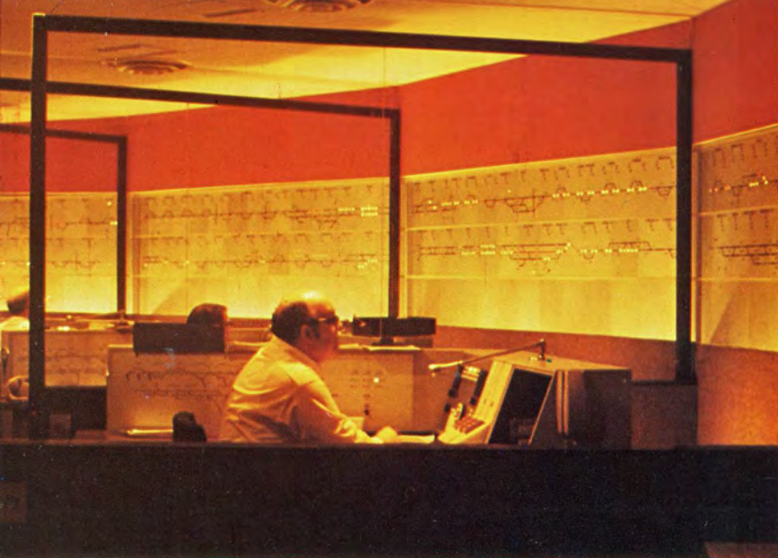
Top: CTC dispatching center in North Little Rock.
